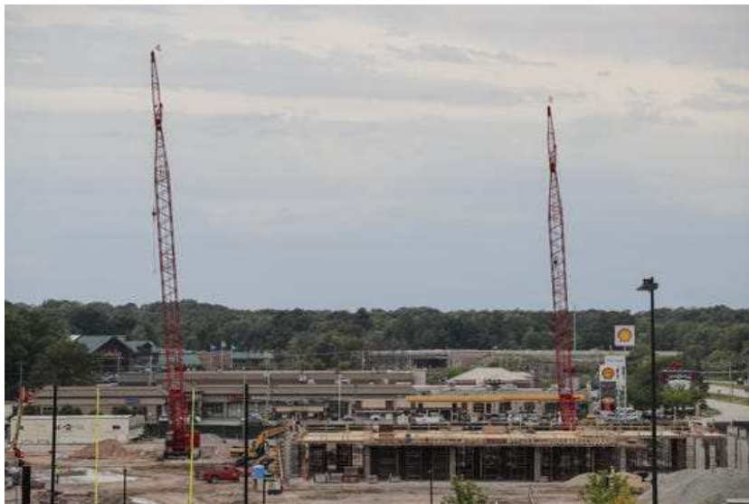
Miron Construction works on the podium project, phase two of Titletown construction, Thursday, September 5, 2019, at west end of Titletown in Ashwaubenon, Wis. (Photo: Joshua Clark/USA TODAY NETWORK-Wisconsin)
