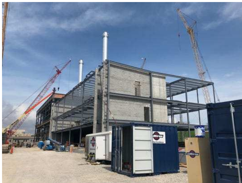
The new Green Bay Packaging mill is beginning to rise in August 2019, roughly one year after Miron Construction began work on the site. (Photo: Courtesy of Miron Construction)
